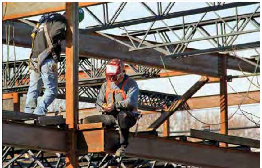
Steelwork rises at the site of the new Mid Coast Medical Group– Bath office on Centre street. The internal medicine group hopes to be in its new quarters by late spring. (Photo by Gerry Maraghy)
